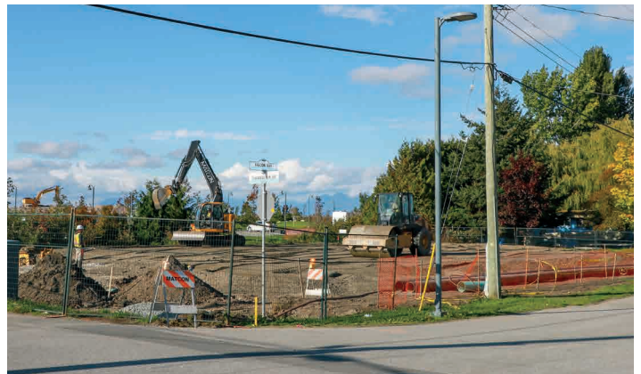
TFN/Matcon has begun work on the ground densification at the new Youth Centre site.
